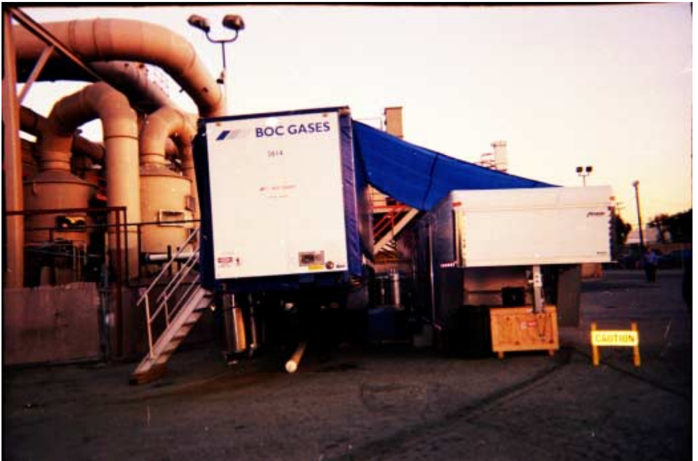
Figure 4 LoTOx System Demonstration Trailer Installation At RSR Quemetco, Inc.
