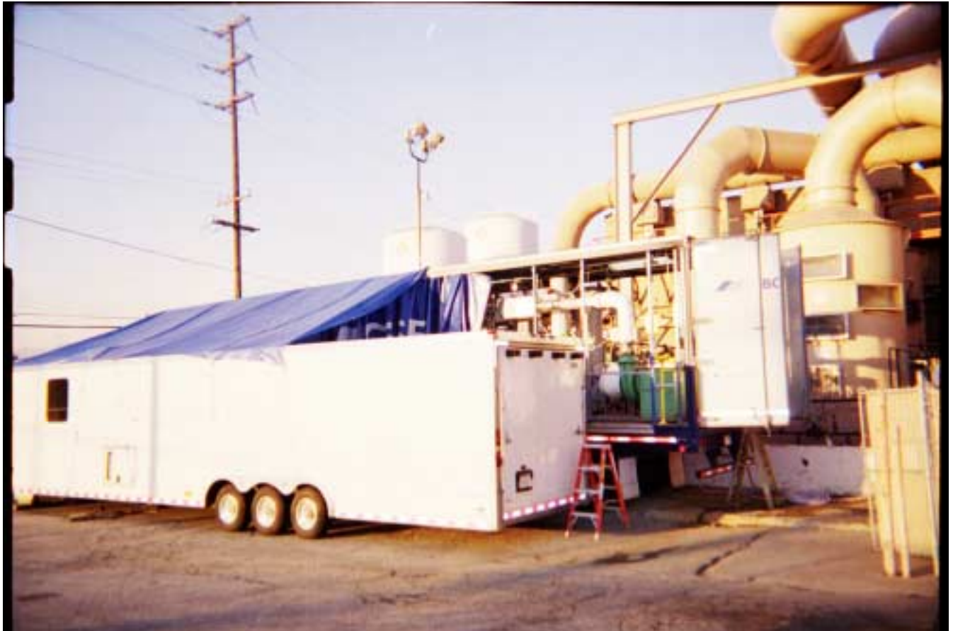
Figure 5 LoTOx System Demonstration Trailer Installation At RSR Quemetco, Inc.
