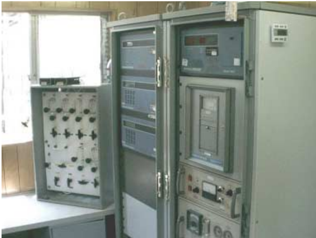
Figure 18. GTI CEM AND TEMPERATURE INSTRUMENTATION INSTALLED INSIDE TRAILER
