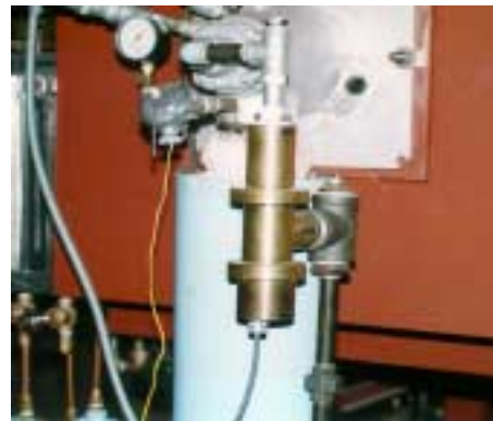
Figure 4. PROTOTYPE CERAMPHYSICS SSP VALVE INSTALLED ON GTI'S TEST FURNACE
