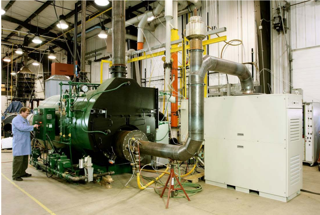
Figure 19. FlexCHP-65 Setup at GTI
