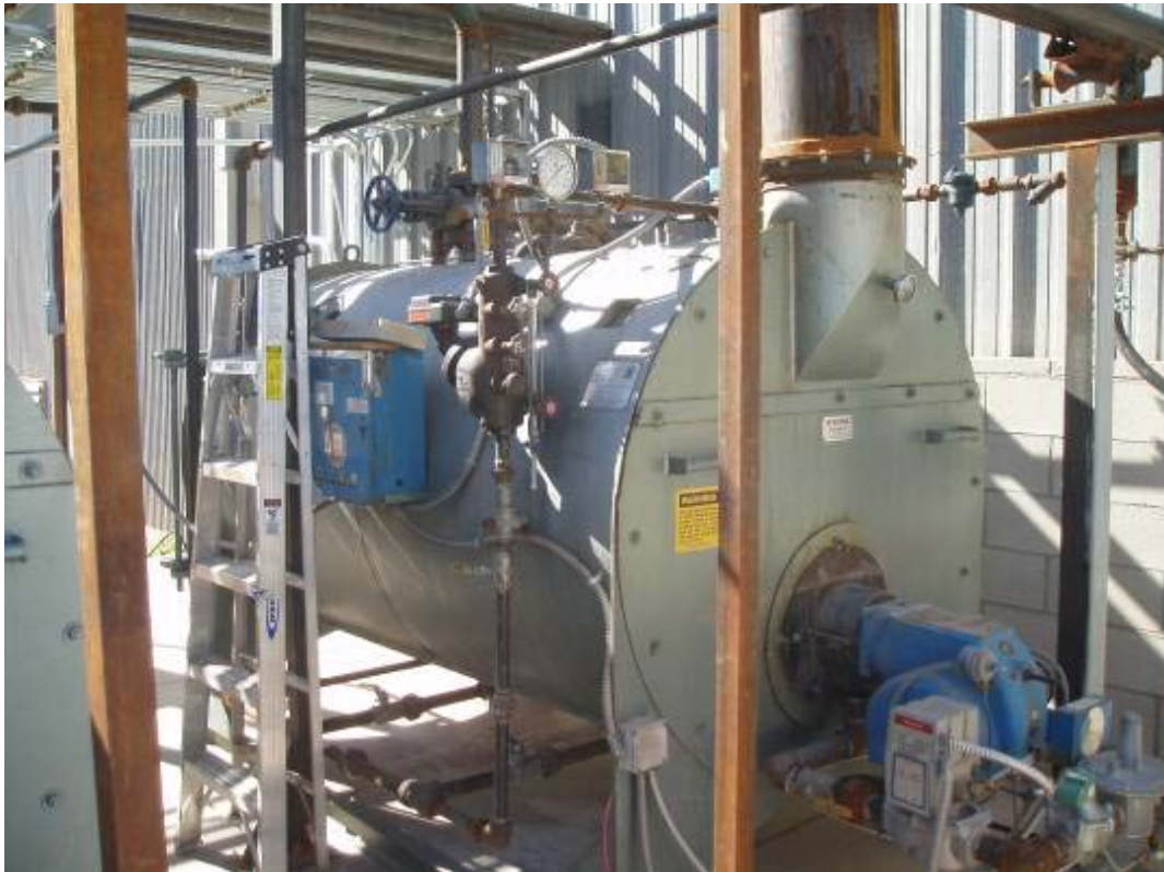
Figure 15. Existing 50 HP Firetube Boilers
