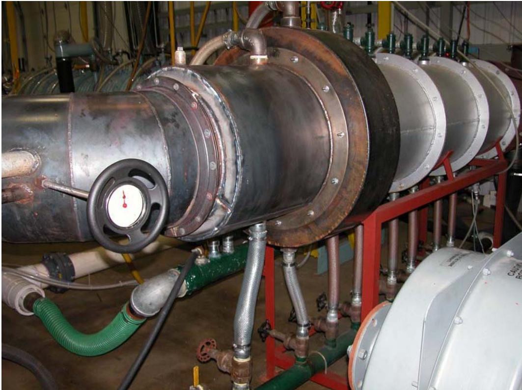
Figure 4. Auxiliary Combustor to Generate STEG
