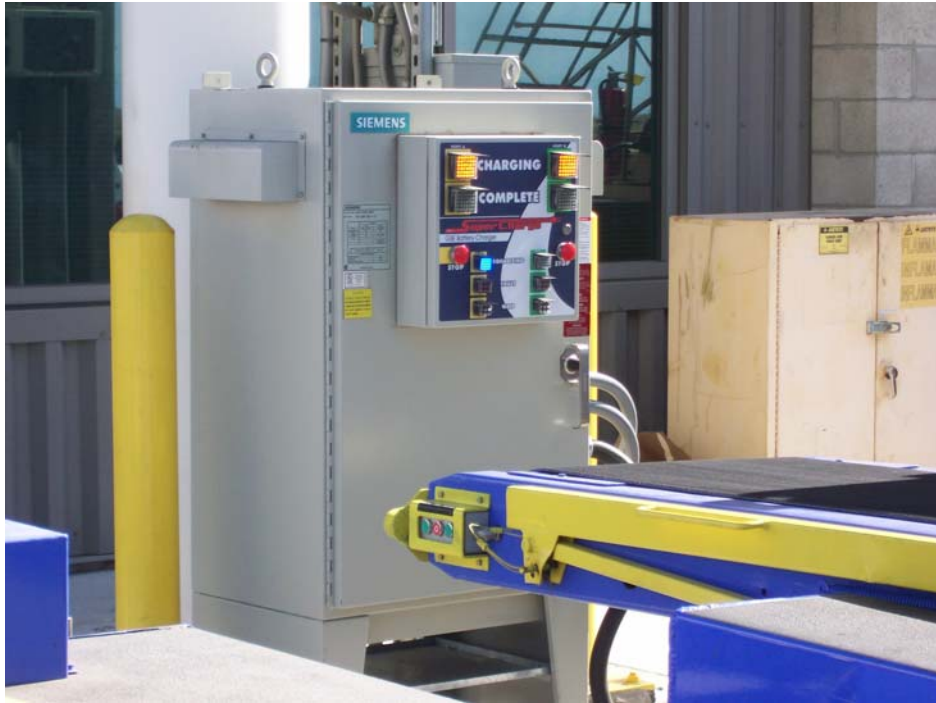
Figure B2—Charger In Service
