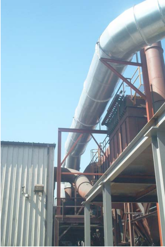
Figure 13 Ductwork Installed to Transport Emissions From Baghouse to Scrubber
