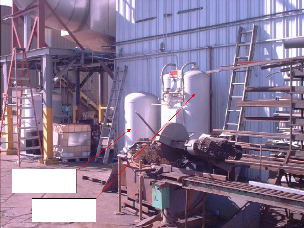
Figure 8 Oxygen Receiving Tank and Oxygen Concentrator. Oxygen Concentration uses Molecular Sieves to Convert Compressed Air into 95+% Pure Oxygen for use in the Ozone Generation Panels
