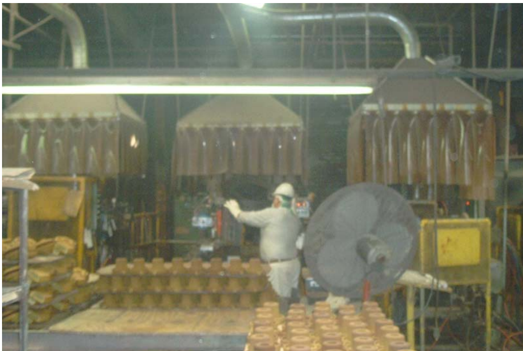
Figure 12 Core Room Emissions Collection System
