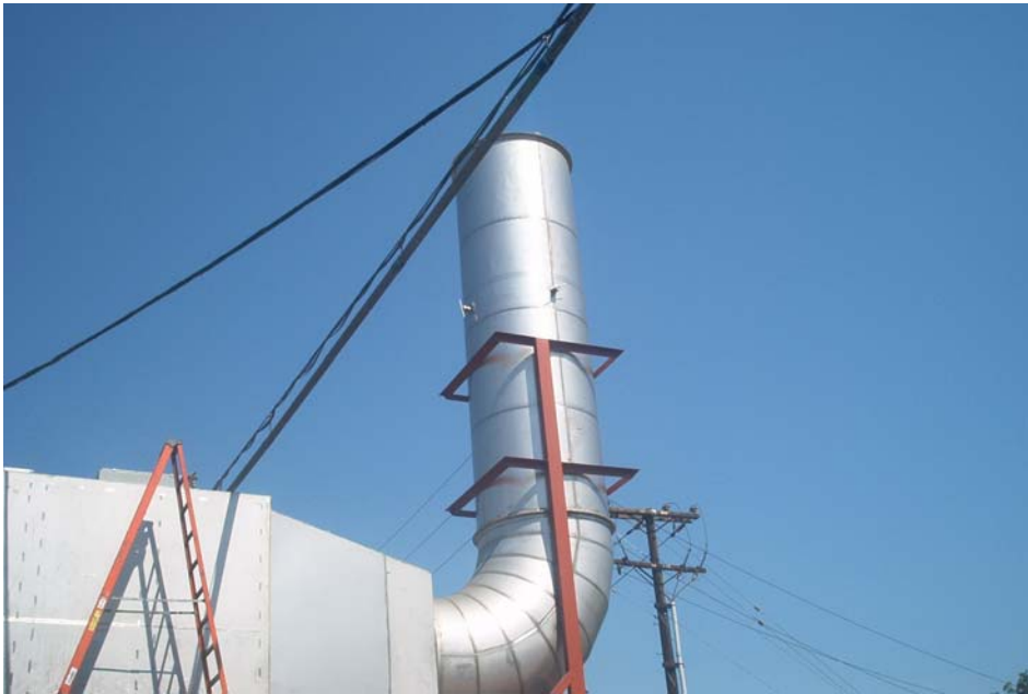
Figure 14 Scrubber Stack with Sampling Ports
