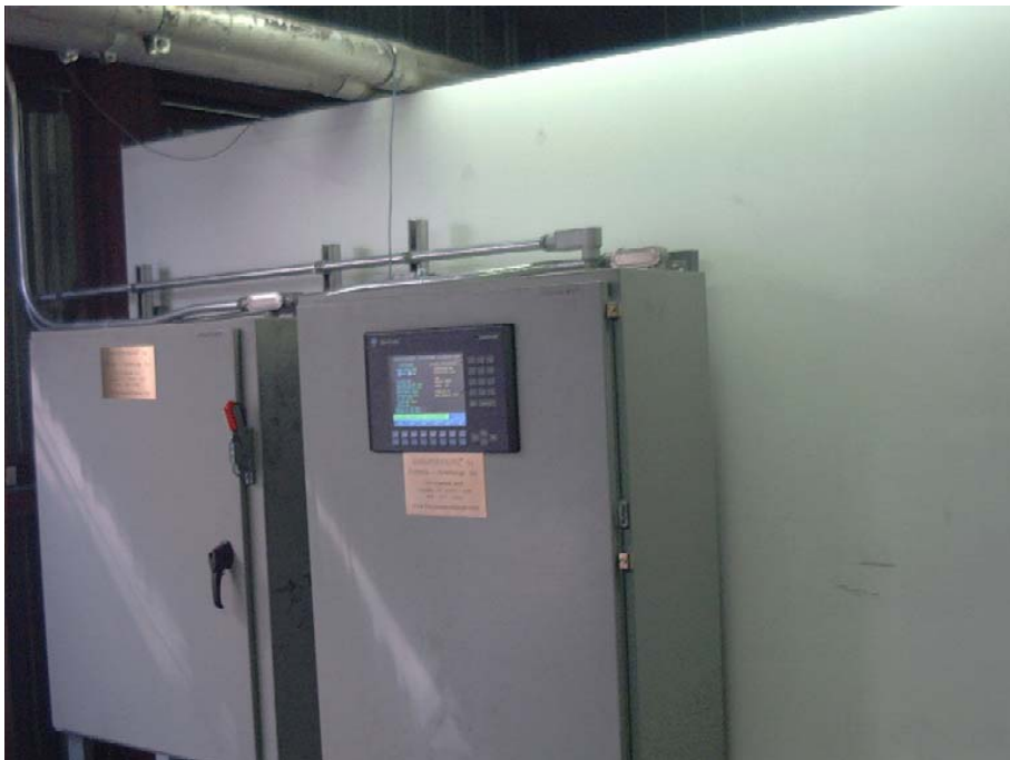
Figure 7 Control and Ultrasonic Panels. Control Panel on Right Monitors and Operates All Systems and Subsystems for Both Scrubber and Blackwater Recycle Equipment. Ultrasonic Panel Contains Power Supplies for the Two Ultrasonic Resonators
