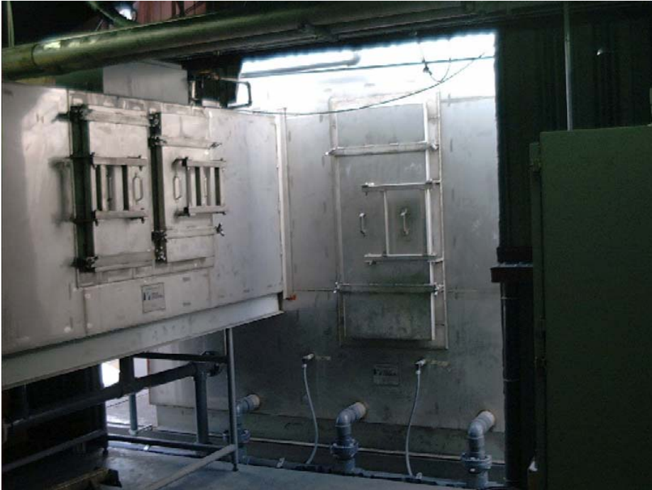
Figure 6 Core Room Scrubber (Left) and its Connection into the Wet Oxidation Plenum (Right). Access Doors Shown for Both Scrubbers Allow for the Replacement of UV Lamps and Scrubber Media Balls
