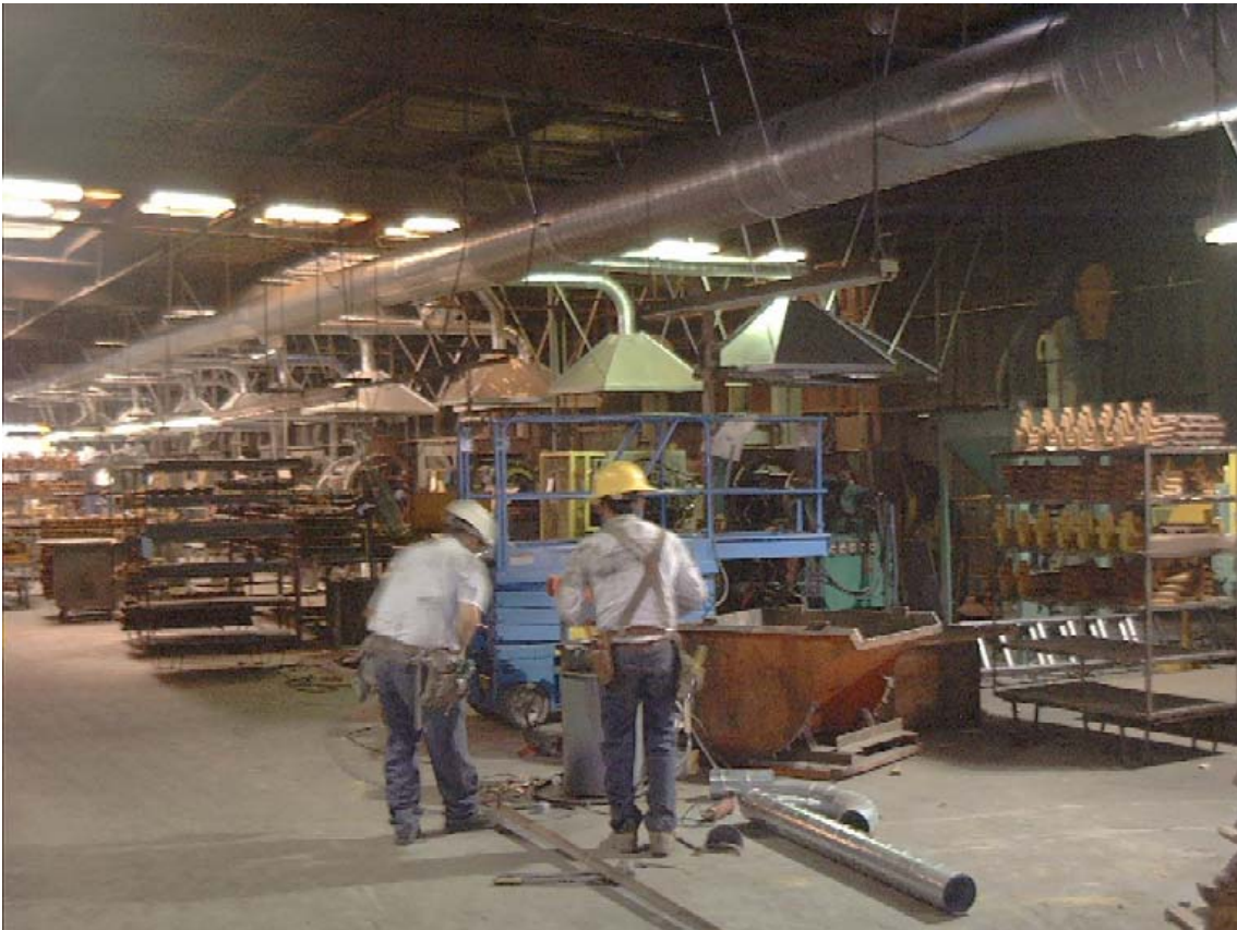
Figure 4 Shell Core Room. Resin Bonded Sands are used for Molding the Interior of the Hollow Castings. New Ducting over Core Molding Machines Installed to Capture Organic Emissions from Resin Binder
