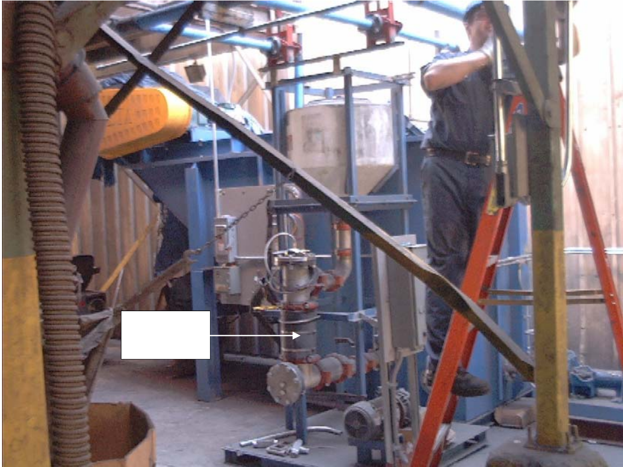
Figure 10 Blackwater System with Acoustic Reactor and Dust Mixing Pump in Foreground
