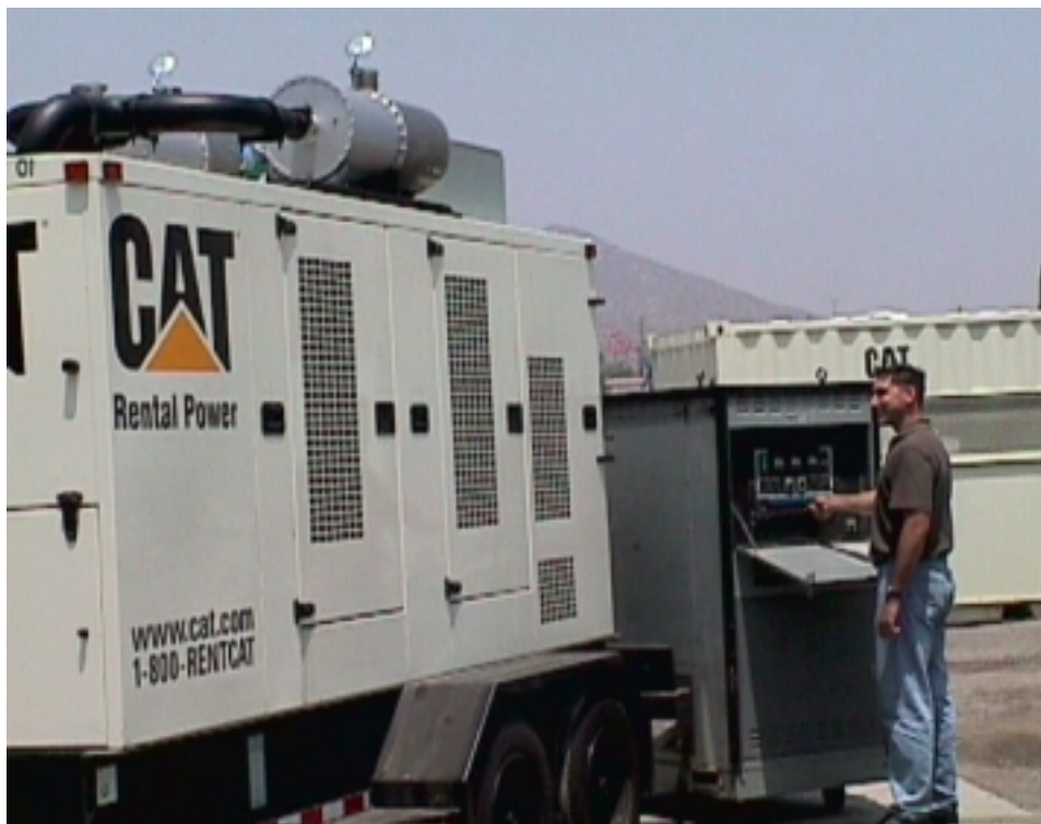
Picture 2: The 225kW installation.
