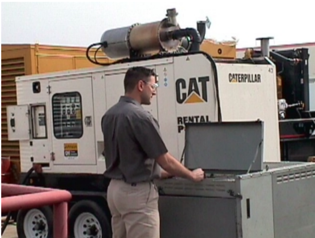
Picture1: The 100 kW installation.
