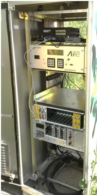
(a) Hardware Deployment at Traffic Monitoring System Cabinet
