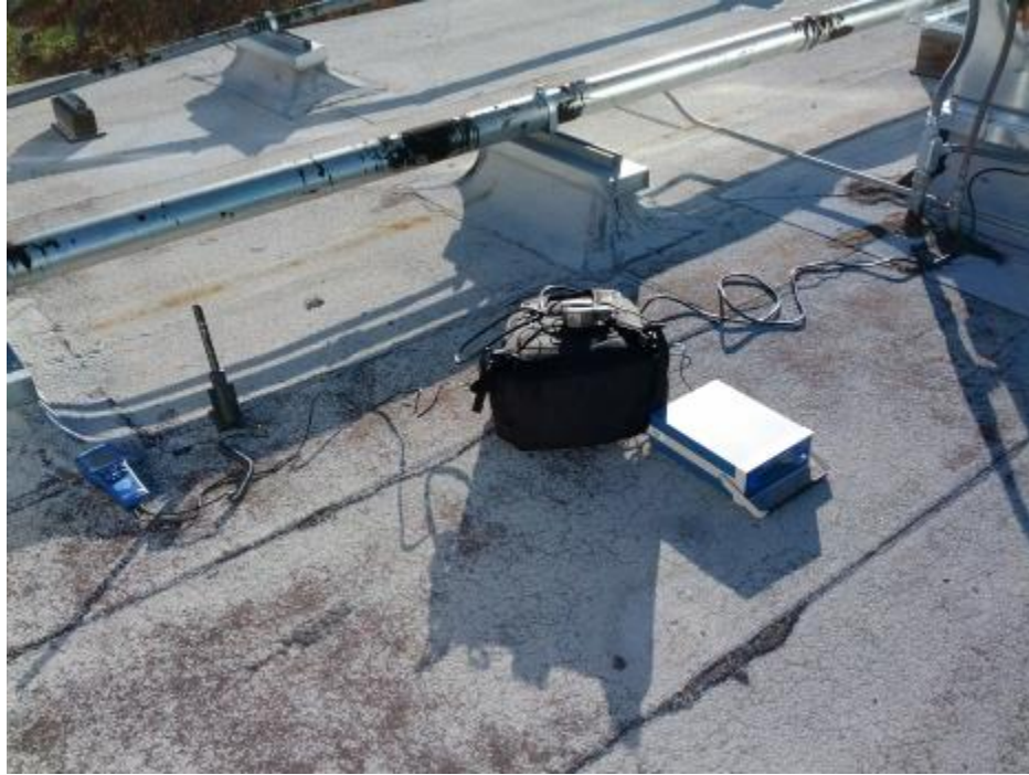
Figure 9.38. Image of outdoor monitoring sit on classroom roof.
