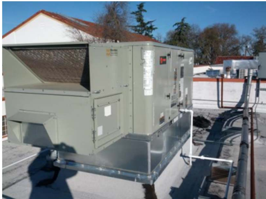
Figure 9.37. Image of TCACS roof-top unit above classroom.
