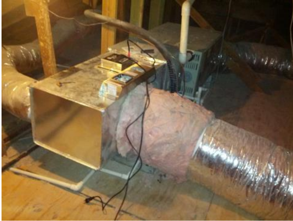
Figure 9.26. Image of HVAC UV 560 and activTek INDUCT 2000 installed after air handler.
