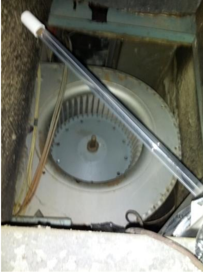
Figure 9.29. Image of HVAC UV 560 installed in plenum after fan.
