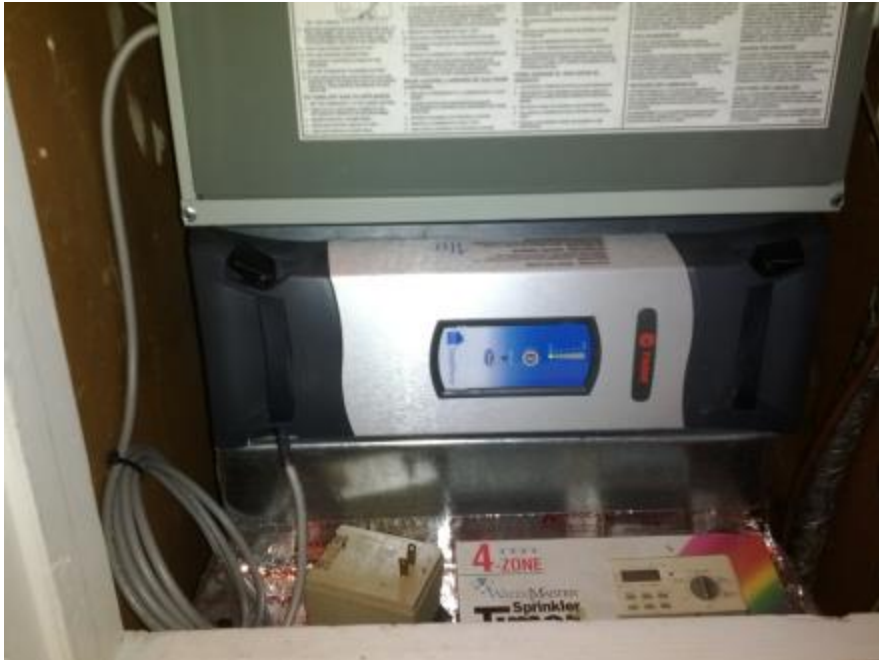
Figure 9.18. Image of device tested (Trane Clean EffectsTrane Clean Effects) as installed in air handling system.
