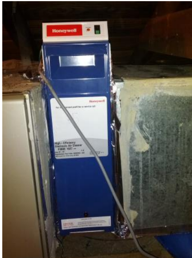
Figure 9.33. Image of Honeywell EP installed.
