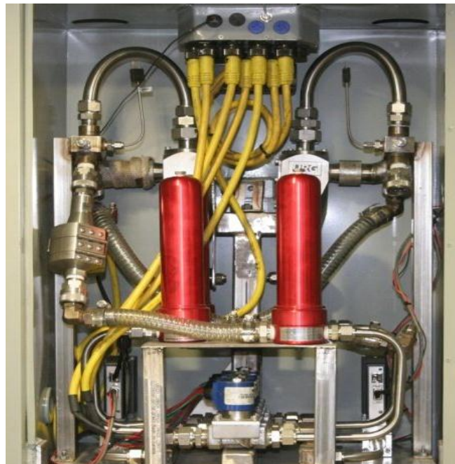
Figure 7 1065 compliant PM sampling system on-board the transportable laboratory container
