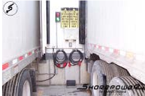
Figure III.A-3: Loading Dock Power Plugs
