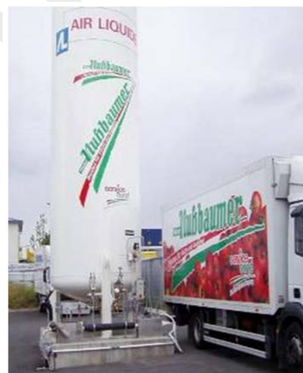
Figure III.E-14: LN 2 Fill Station (Air Liquide, 2009)
