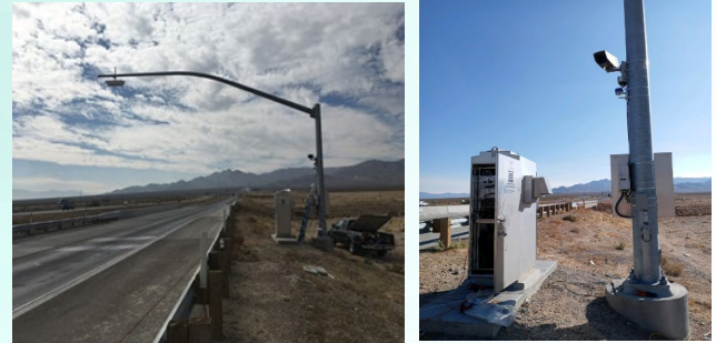
Cameras installed near Mountain Pass
