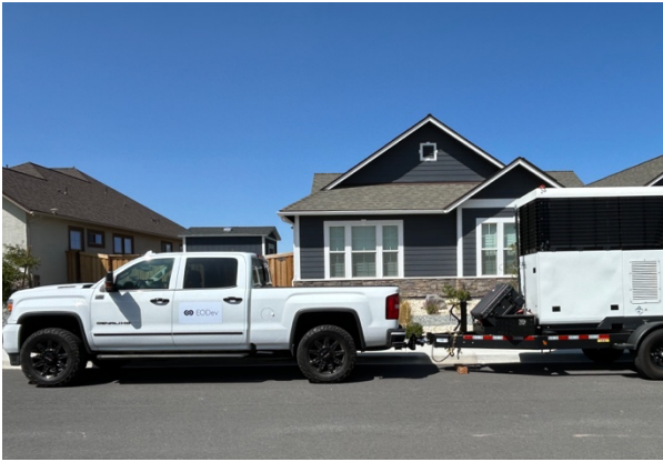
Figure 6. Typical transportation configuration for a portable diesel power generator during field deployment.
