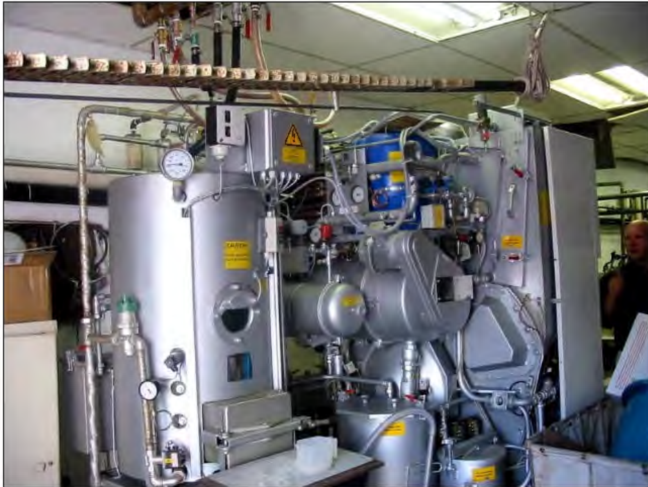
Figure 1: Image depicting dry cleaning solvent tank and distillation system.
