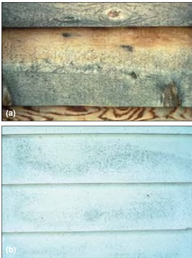
Figure 16–24. Mildew is most common in shaded, moist, or protected areas (a) on wood and (b) on painted wood.
