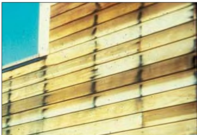
Figure 16-28. Iron stain on newly installed wood siding. Poor quality galvanized nails corrode easily and, like uncoated steel nails, usually cause unsightly staining of the wood.
