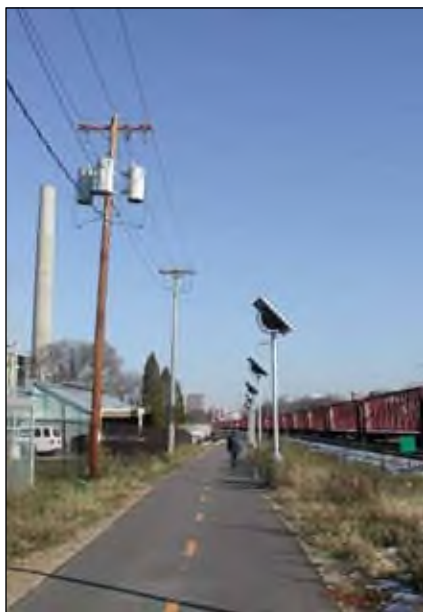
Figure 6–4. An example of round timber poles used for electrical utility distribution.
