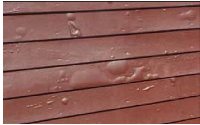
Figure 16–21. Water blisters (also called moisture blisters) caused bubble-like deformation of paint film.
