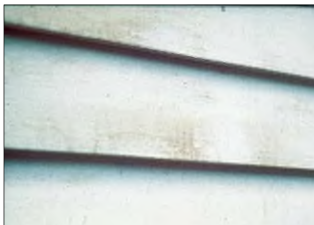
Figure 16–25. High moisture content of wood can cause diffuse extractives bleed, particularly if a stain-blocking primer is not used.
