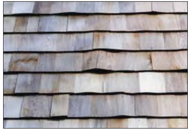
Figure 16–17. Shingles installed with insufficient gap later warped when they expanded after getting wet.
