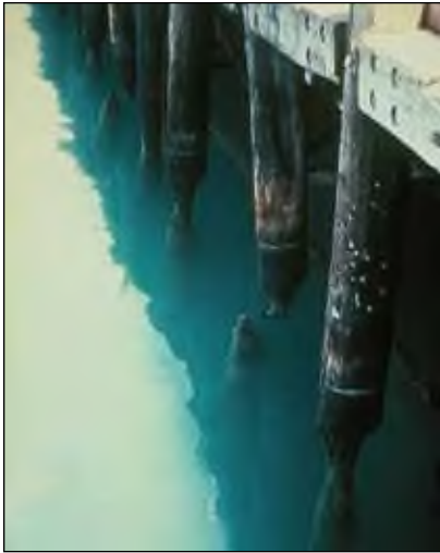
Figure 14–11. Limnoria damage to piling.
