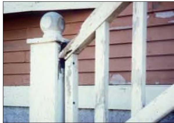
Figure 16-14. Decay and paint failure in wood railing fully exposed to weather.
