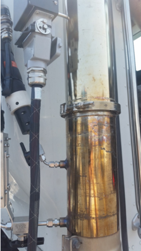
Figure 5. Exhaust pipe with sampling pores on a vertical type exhaust
