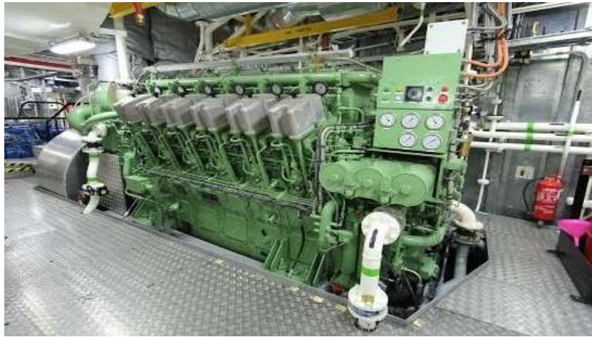
Figure H-3. Tugboat Engine Room with 3,600 Horsepower Main Engine
