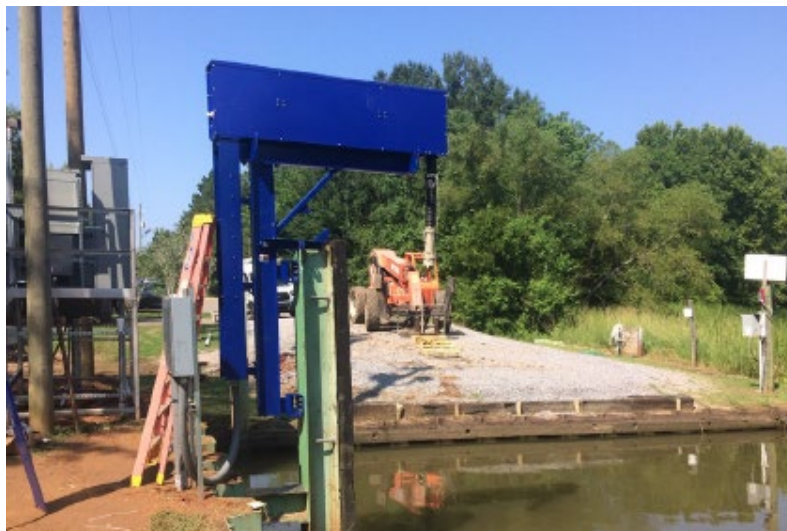
Figure E-46. Gee's Bend Ferry Dock Charging Station 243
