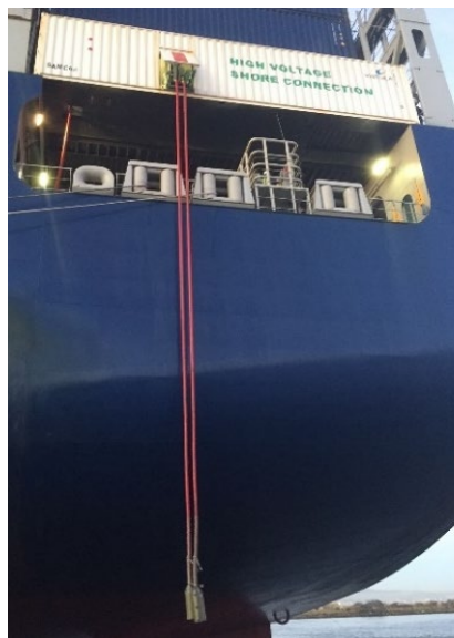
Figure I-21: Vessel Side Shore Power
