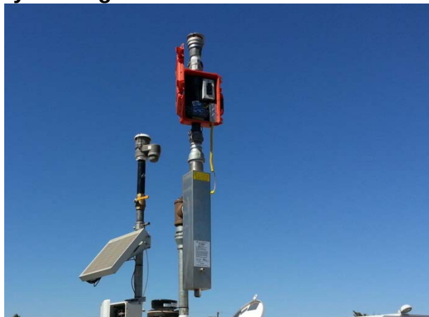
PV-Zero Installed on Vent Line
