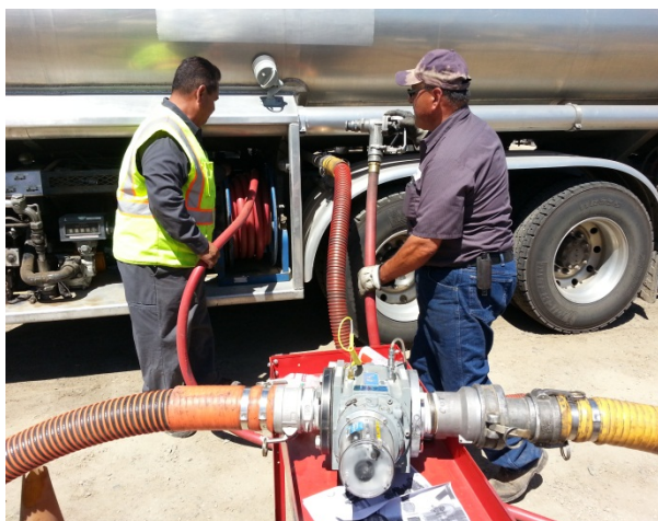
Volume Meter Installed on Vapor Return
