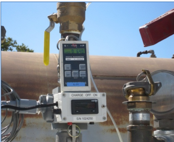
Manometer Installed on Vent Line
