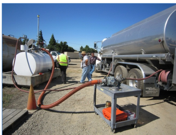
Product and Vapor Lines During Delivery
