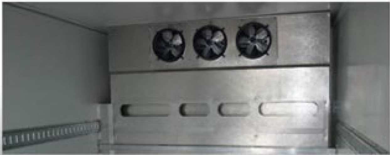
Figure IX-3. Cold Plates and Blowers
