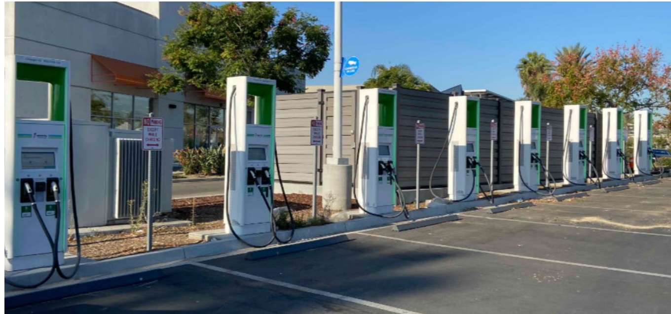
Legacy chargers before upgrades
