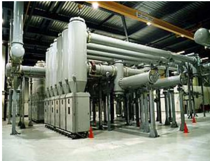
SF 6 Gas Insulated Substation Source: CARB
