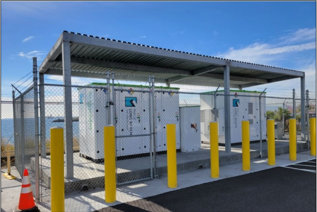
Figure 42: Battery-Electric Storage System at Port of Long Beach 118
