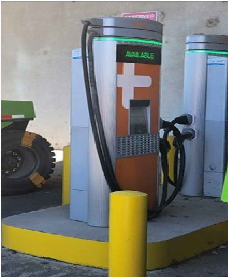
Figure 44: Battery-Electric CHE Charging Station (Staff photo)
