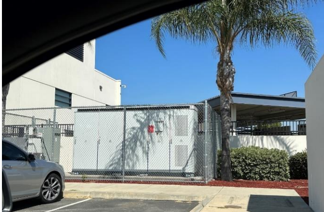
FIGURE 8: ENGIE BATTERY ENERGY STORAGE SYSTEM
