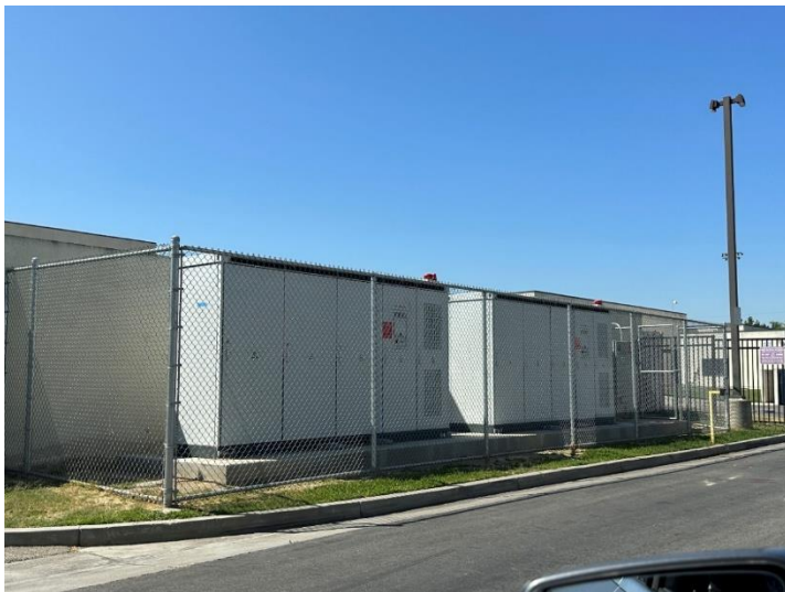
FIGURE 9: ENGIE'S BATTERY ENERGY STORAGE SOLUTION
