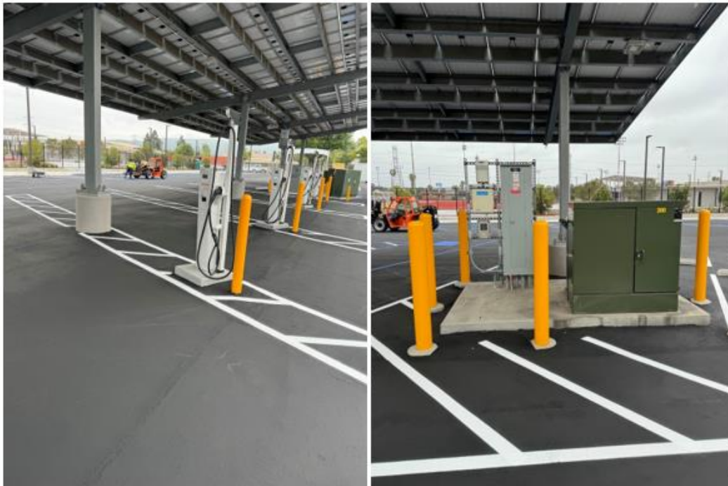
FIGURE 7: CHARGING STATIONS AT MT.VIEW HIGH SCHOOL
