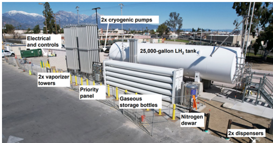
Figure 47. Example hydrogen fueling station at Foothill Transit.
