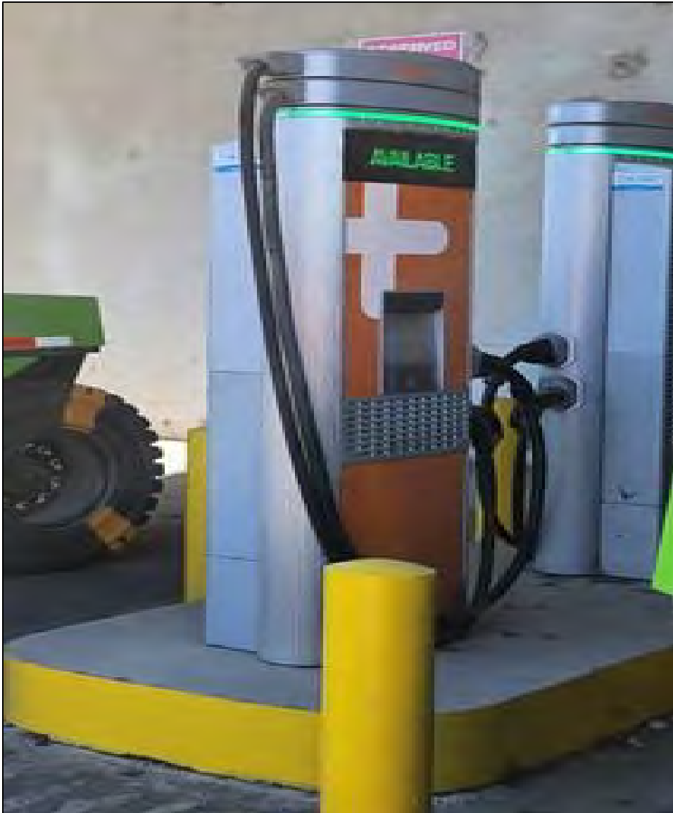
Figure 44: Battery-Electric CHE Charging Station (Staff photo)
