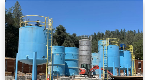
Fortera Redding ReCarb® Commercial Plant Development
