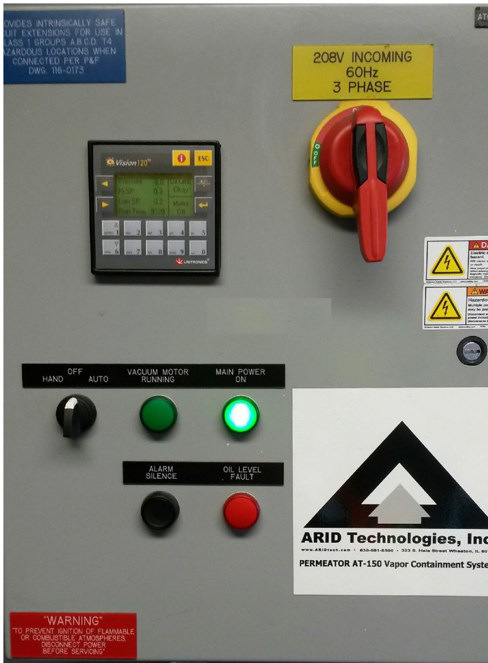
FIGURE 8-2 Configuration of Permeator Control Panel Hand/Off/Auto Control Knob in OFF position to Conduct TP-201.3
