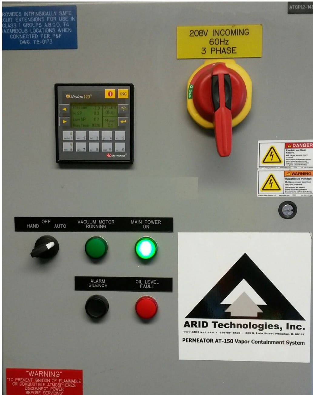
FIGURE 8-3 Configuration of Permeator Control Panel Hand/Off/Auto Control Knob in AUTO position after Conducting TP-201.3
