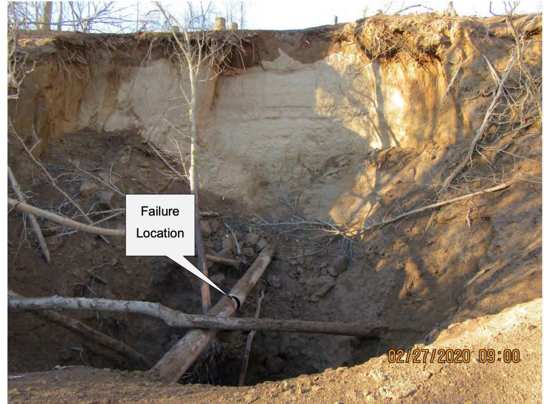
Figure 6. Failure Location (Upstream to Downstream)
