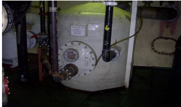
Figure 33. The Sludge Tank
