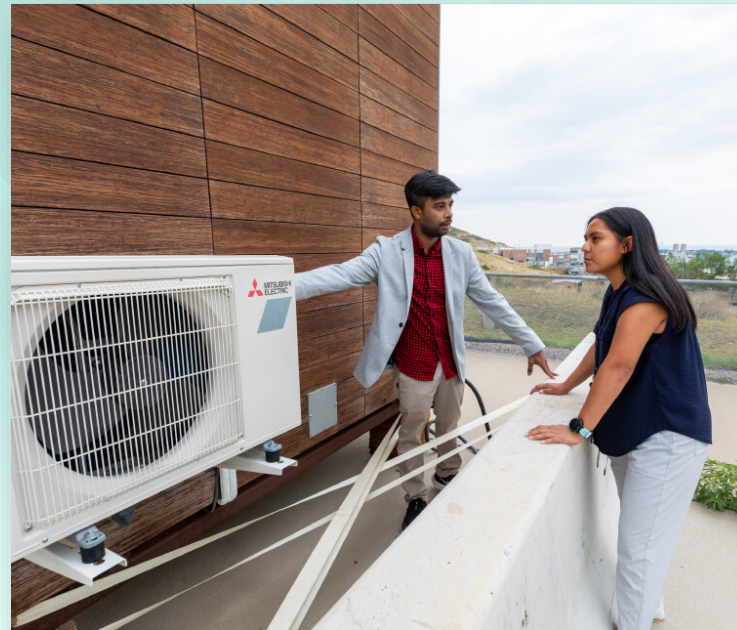
Photo by Werner Slocum / NREL
