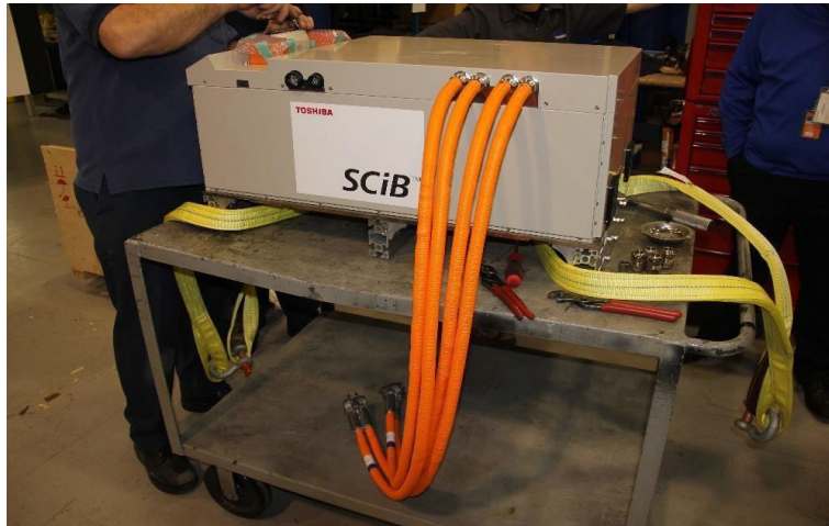
Figure 7. High-Voltage Battery Assembly
