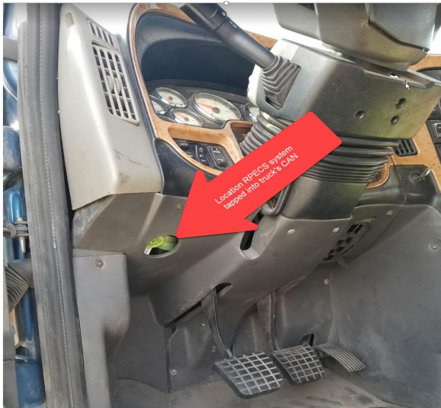
Figure 17. Location that RPECS Datalogger Tapped into the Diesel Fueled Truck's CAN Port
