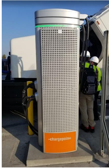
Figure 12. Electric Drayage Truck Charging Station
