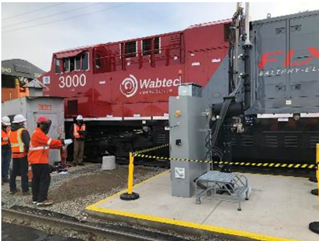
Figure 8. Image of BEL While Charging at the BNSF Stockton Momorn Yard
