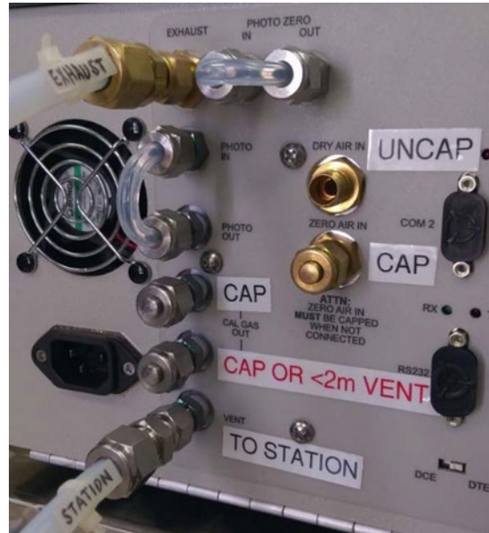
Figure 4: Example Tubing Configuration for Station Manifold Connection - 3/8" OD Tubing with Vent Port Capped
