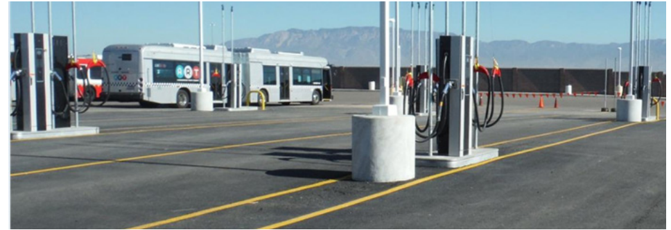
Figure 3-1. A Plug-in Charging Yard | Source: WSP
