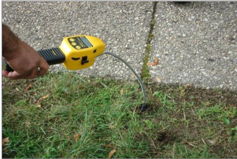
Figure 4 – The CGI meter used to identify the leak area
