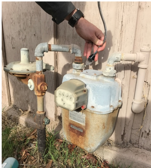
Figure 6 – The CGI used to identify the leak
