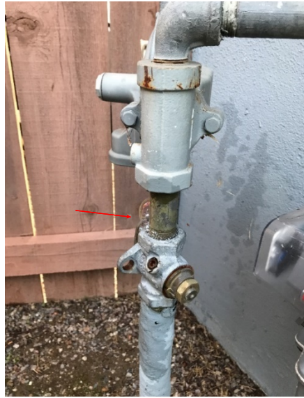
Figure 7 – Example of Soap Bubbles on Leaking Valve
