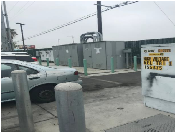
LADWP Transformer and Main Switchgear
