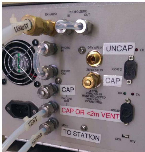
Figure 2: Example tubing configuration for presentation to the station's sample manifold using a length of ¼" OD Teflon tube. In this example, venting of bypass flow is accomplished through a second length of ¼" OD Teflon tubing connected to the "Vent" port of the transfer standard.
