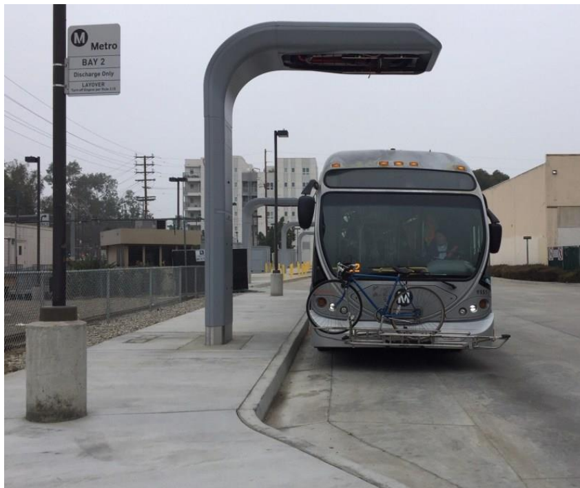
Figure 4-4. North Hollywood Station On-Route Charger
