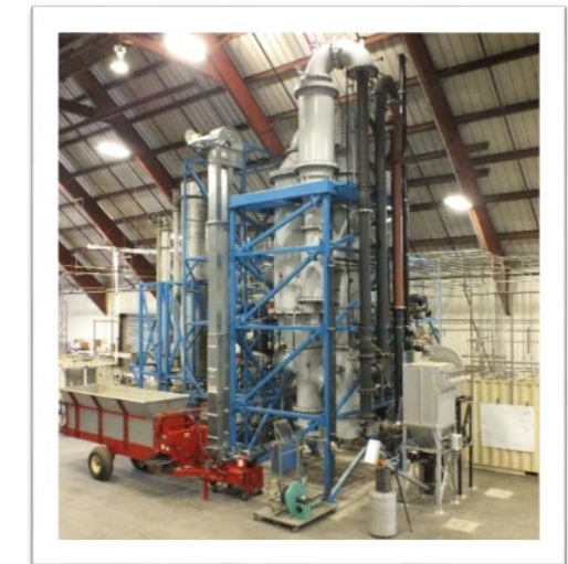
Photo of the fast internally circulating fluidized bed gasifier at the Woodland Biomass Research Center
