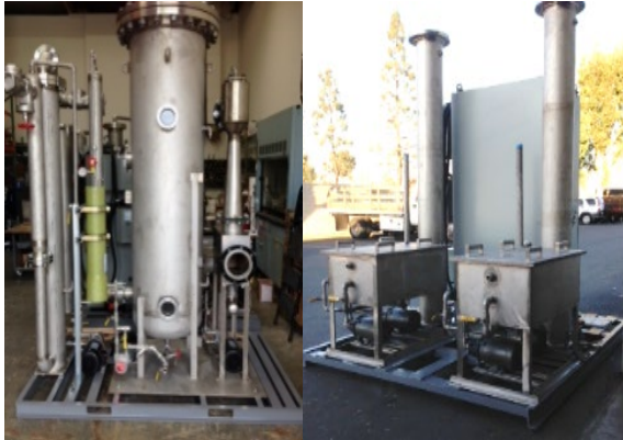
Skid-mounted subsystem to convert landfill gas to RG via a novel cleanup and upgrading technologies.
