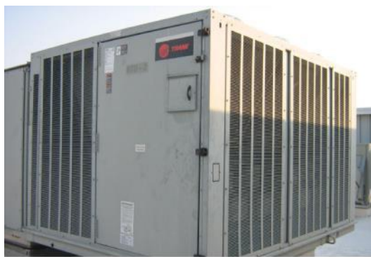
Rooftop HVAC system
