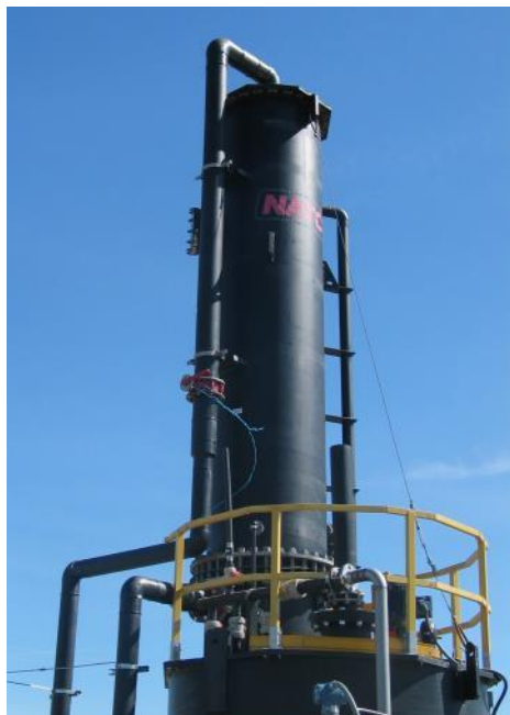
Dairy gas cleanup system (gas scrubber)
