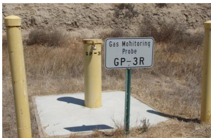
Gas monitoring probe at an unnamed state landfill.
