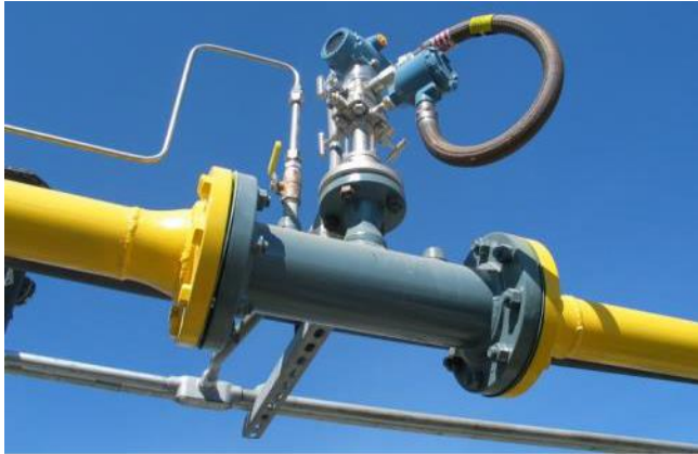
Gas flow meter for natural gas made at a dairy digester
