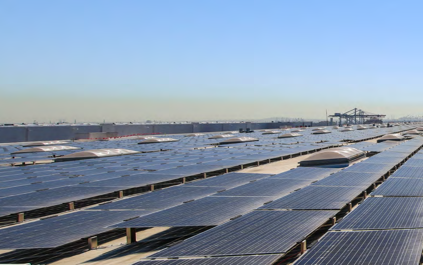
Rooftop solar installation at the Port of Los Angeles. Office of Mayor Eric Garcetti (CC BY-NC-ND 2.0)
