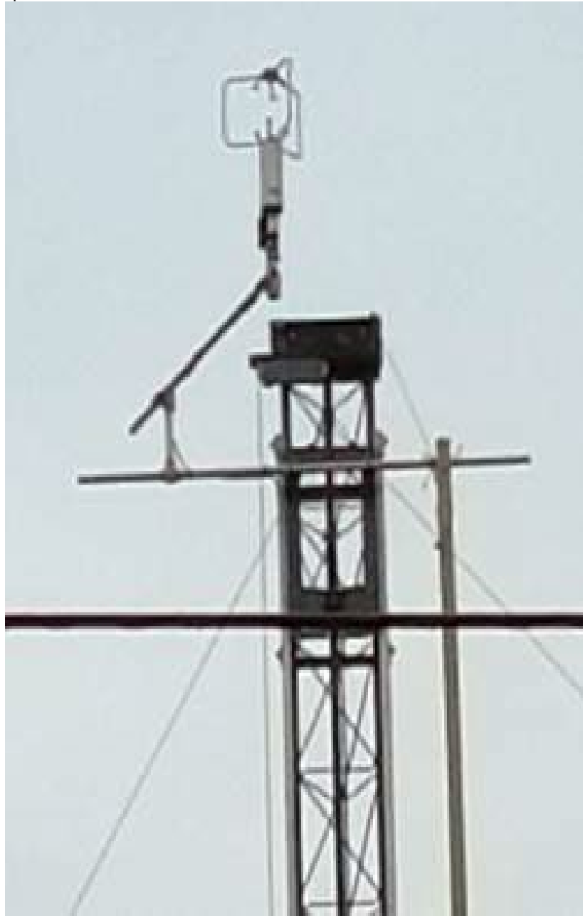
Figure 2: Sensor Installation View
