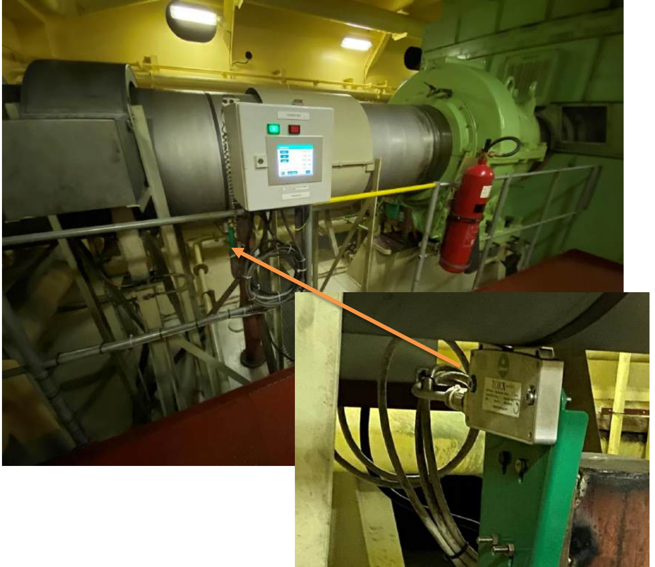
Figure D-5 ME instrumented drive shaft and strain gaguge measurment system
