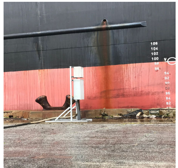
Terminal 3 had 480V/400A shore power available for docked vessels.
