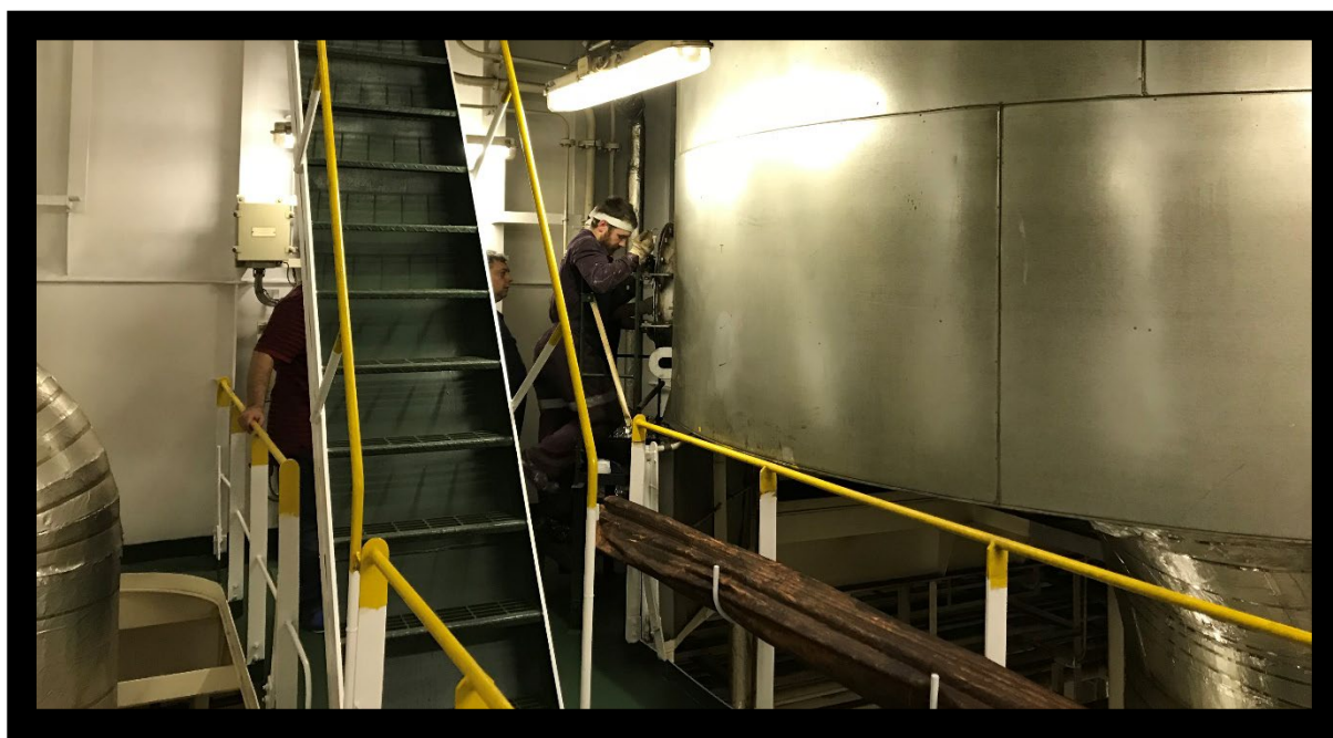
Figure 2-2 Setup on the ME, before the economizer (two decks above the ME)
