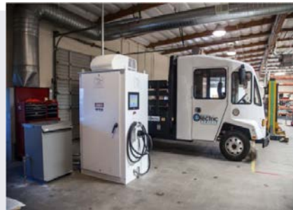
Standardized charging infrastructure
